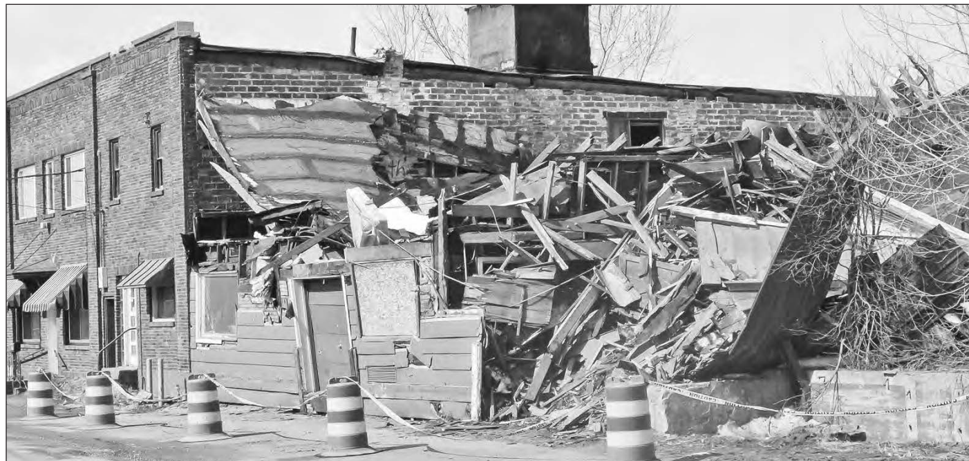
THE CITY of Ironwood has secured grant funding to help fight blight within the city limits, including the removal of the property at 238 E. Ayer Street, seen Wednesday, that collapsed under the weight of the snow load this winter.
